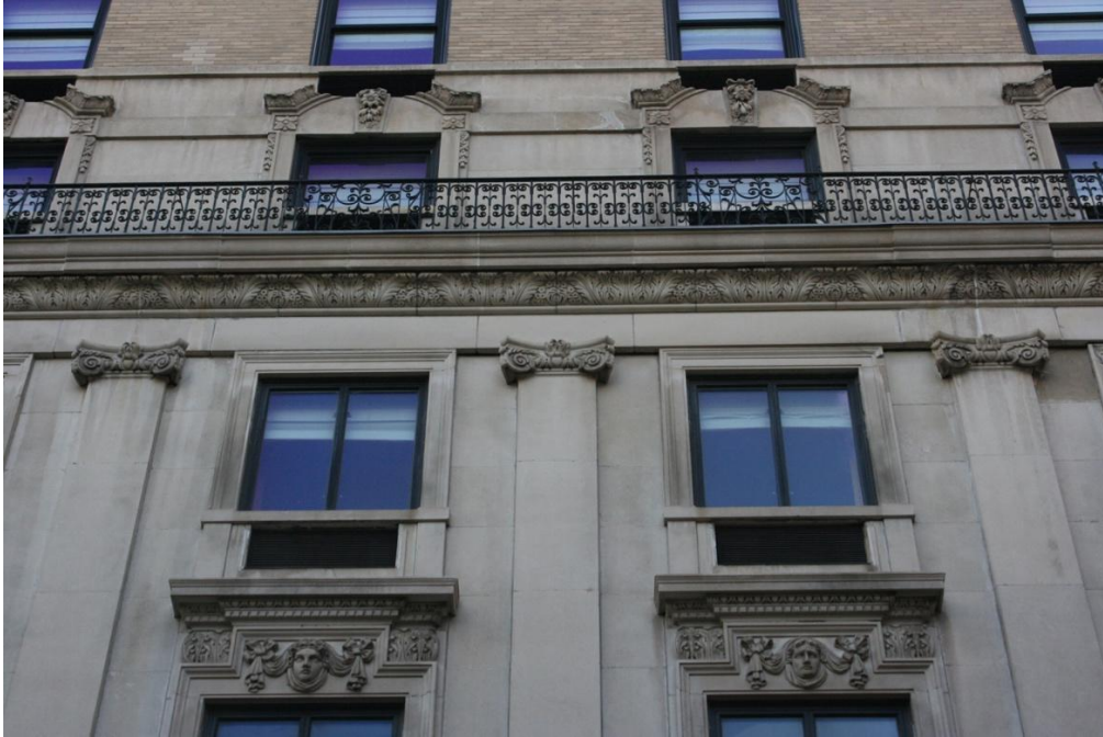
Figure 9. School Street façade; detail of trim at third, fourth, and fifth floors. July 2020.
